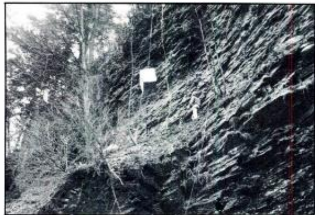
Figure 5. During the precarious installation, 160 lb. speakers were hoisted and positioned within the 110-foot cliffs of the Gorge.
