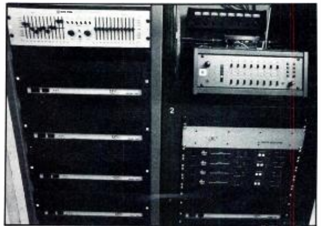
Figure 4. A portion of the audio rack designed by PRS Service Department.
